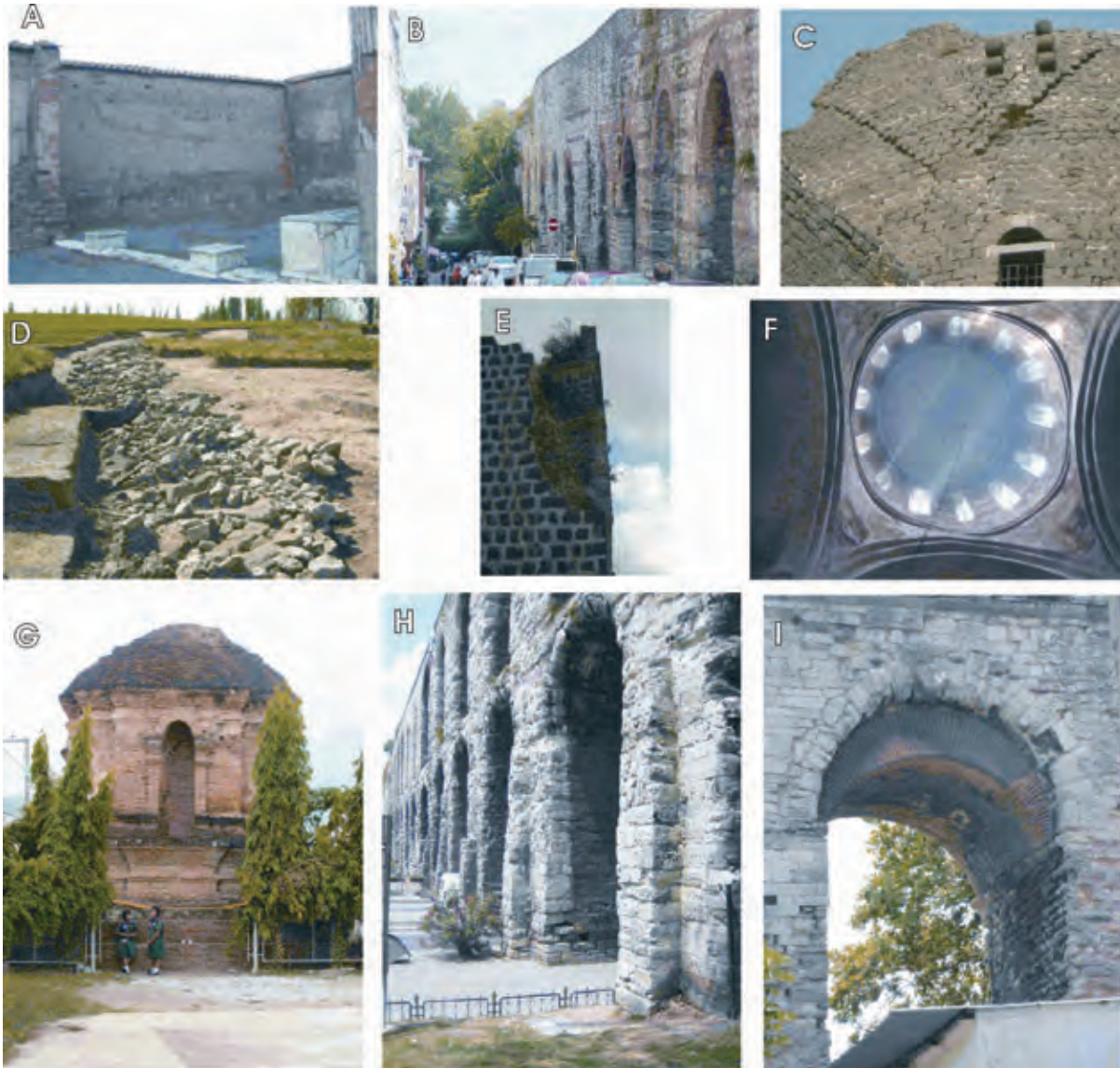
Figure 2: A. Arcuate out-of-plane collapse in the market, Pompeii, Italy, repaired before the 79 AD eruption of Vesuvius, which buried the city. Photo: Kázmér #9266. B. Warped northern side of the Valens aqueduct (Istanbul, Turkey). Completed in 368 AD, several subsequent earthquakes left their traces on the massive construction #0340. C. V-shaped damage on the SW wall of the twelfth-century donjon of al-Marqab citadel, coastal Syria. The damage was inflicted by the 1202 earthquake (Kázmér and Major, 2010) #4589. D. Fallen masonry fence in the Roman city of Carnuntum (Deutsch-Altenburg, Austria) #5496. E. Triangular missing parts in corners of walls (al-Marqab citadel, coastal Syria) #4671. F. Deformed circular dome of fourth- to eleventh-century Samtavro cathedral, Mtskheta, Georgia #1633. G. Tilted Buddhist stupa (approximately fifteenth century) in Chiang Mai, Thailand. While a single tilted building does not indicate seismic origin, this stupa is one of 21 sites displaying tilting in the city (Kázmér et al. 2011) #3411. H. Buttresses support the pillars of the Valens aqueduct in Istanbul, Turkey, completed in 368 AD #0335. I. Valens aqueduct in Istanbul, completed in 368 AD. A brick arch was built to support the weakened stone arch after one of the frequent earthquakes in the region (Istanbul, Turkey) #0335.
