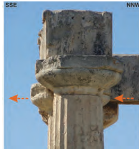
Figure 7: The capital of the column under the restored epistyle that preserves a displacement of ~ 10 cm towards the SSE.
