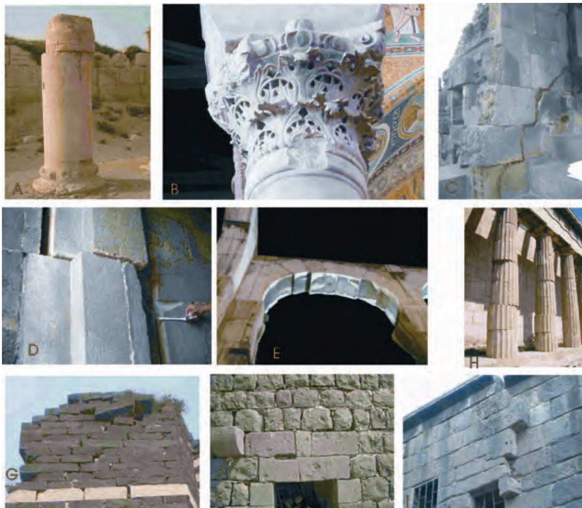
Figure 1: Typology of earthquake-induced damages in ancient buildings. A. Cracks / fractures within a block (2nd century AD Palmyra theatre, Syria). Photo Kázmér #4281. B. Chipped edges of column and capital in the sixth-century Eufraasius cathedral, (Poreč, Croatia), damaged by the 1440 earthquake. #0080. C. Through-cutting fractures (repaired) in the 8-9th century Brahma temple of the Prambanan complex, Yogyakarta, Indonesia, caused by the 2006 earthquake. #6488. D. Horizontal shift of large ashlars; vertical joints opened up between them. Shiva temple, Prambanan complex, Yogyakarta, Indonesia. Tape measure extended 20 cm. #6498. E. Dropped ashlars in a Roman arch (Damascus, Syria). #2017. F. Broken lintels in 12th century al-Marqab citadel, coastal Syria. #4663. G. Clockwise rotated blocks in 12th century al-Marqab citadel, coastal Syria. #5168. H. Displaced drums of masonry columns of the 5th century BC Hephaisteion temple, Athens, Greece. #1132. I. Extruded portion of house wall. Bosra, Syria. #4183.
