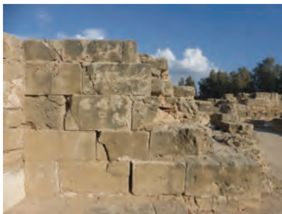
Figure 6: Paphos, Cyprus. Saranda Kolones Crusader castle. Internal pilaster with penetrative fractures.
