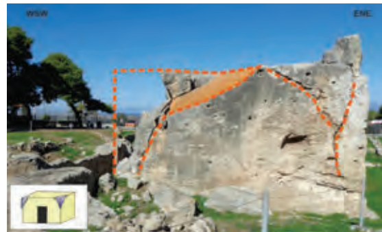
Figure 4: The Glauke Fountain with partial collapse that preserves V-shaped corner cracks at its SSE façade.
