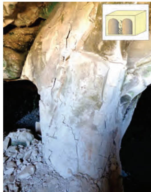
Figure 5: The NE tunnels of Peirene Fountain that preserve crashing/spalling effects on their rock-hewn tunnel wall.
